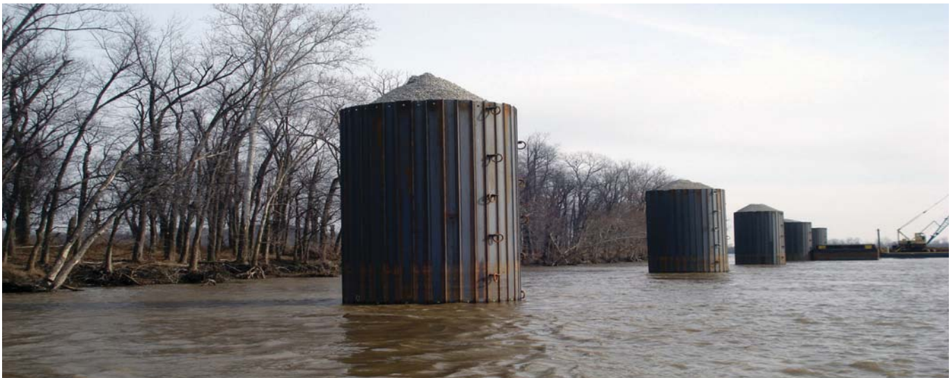
Sitrans Coal Transfer Facility, Mount Vernon, IN
